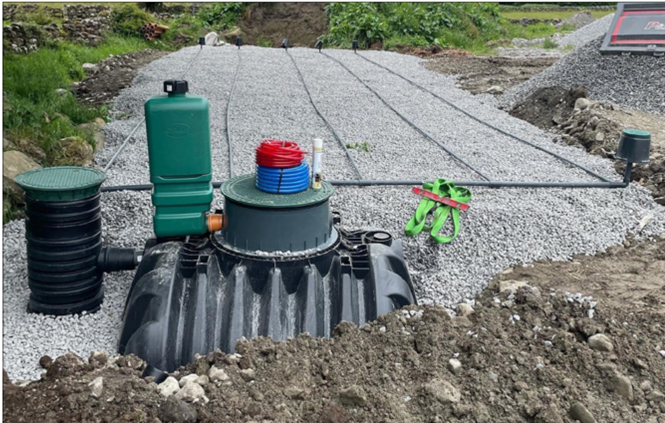
7PE one2clean with 90 m 2 Low-pressure pipe network in Co. Galway.
