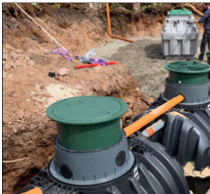
10PE one2Clean with pumped outlet, Co. Mayo.
